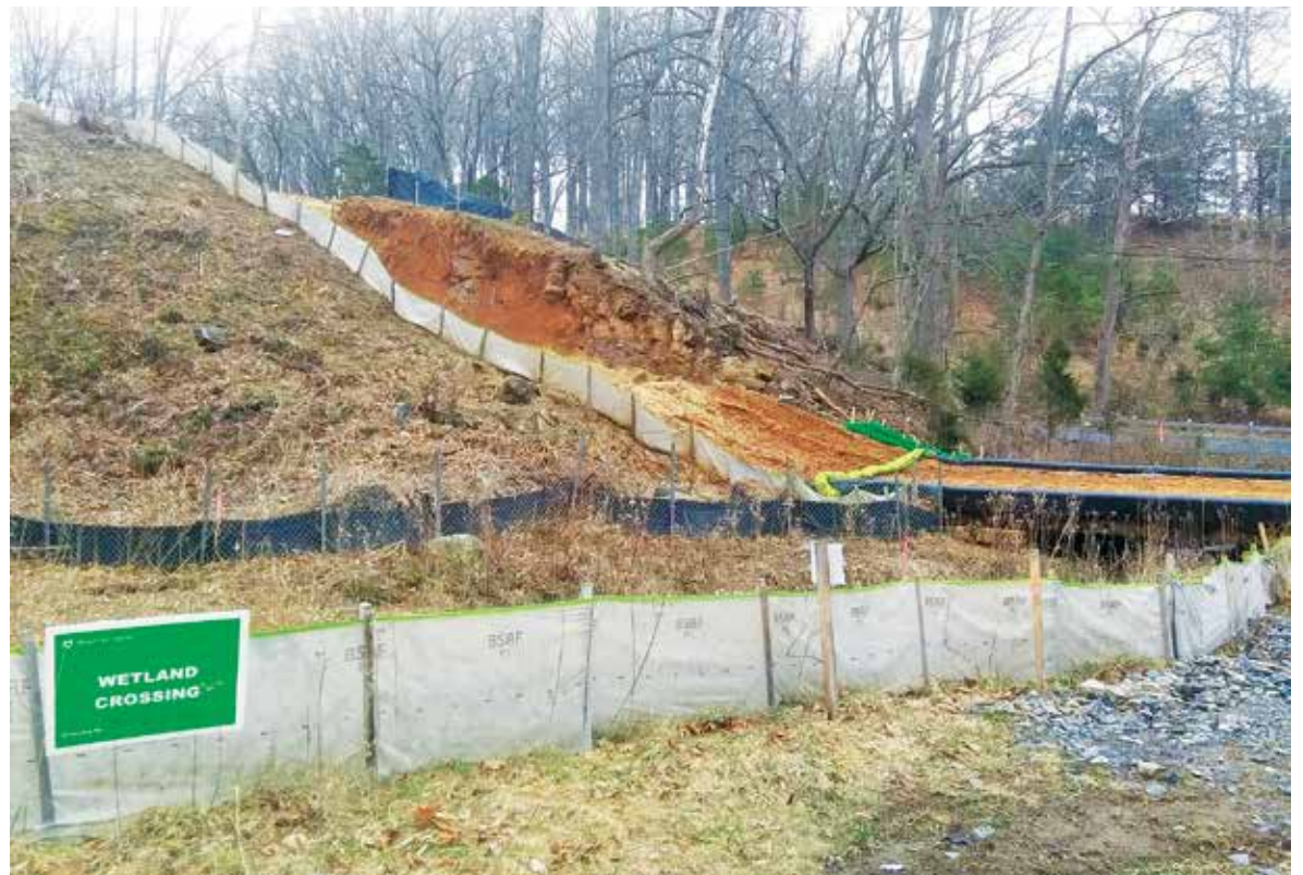
An example of the blatant disregard for forests and wetlands by corporations building the Mountain Valley Pipeline.
