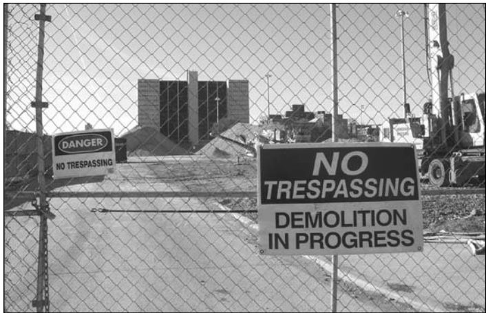
All of the Cabrini Green high-rises are now in the process of being torn down by private contractors.
