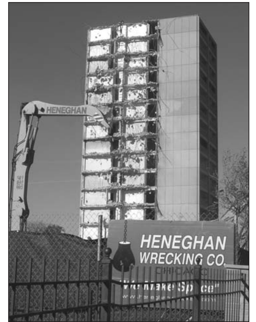
Private contractors tearing down public housing units at Cabrini Green Projects in Chicago.
